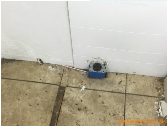
Kitchen range receptacle
