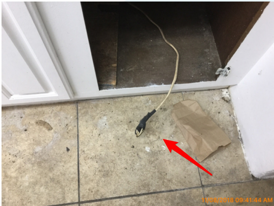
Improperly terminated wire southwest kitchen cabinetry
