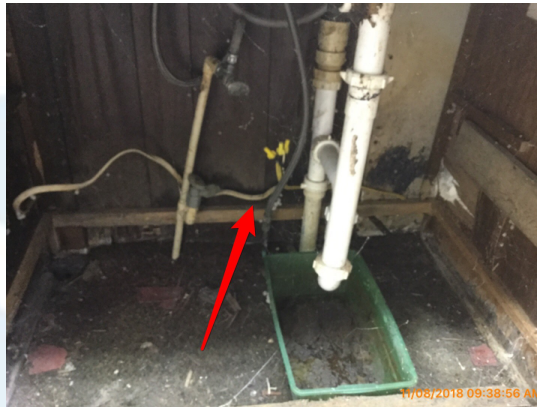
Exposed Romex under kitchen sink.
