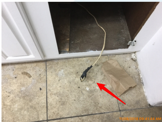
Improperly terminated wire southwest kitchen cabinetry
