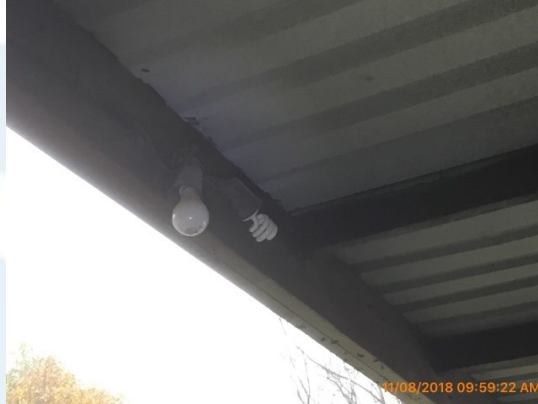
Light at the carport
