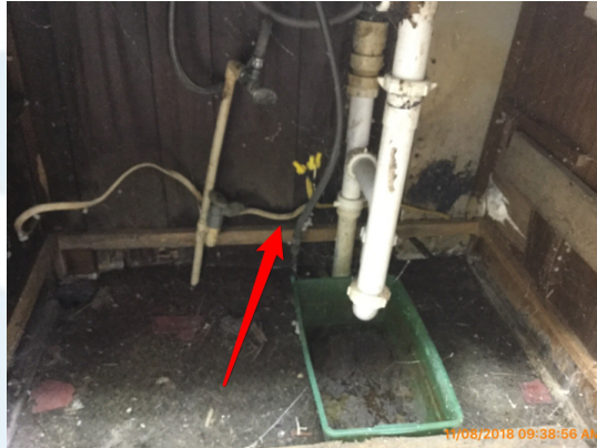
Exposed Romex under kitchen sink.
