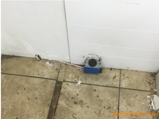
Kitchen range receptacle
