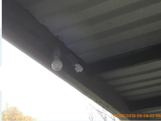
Light at the carport
